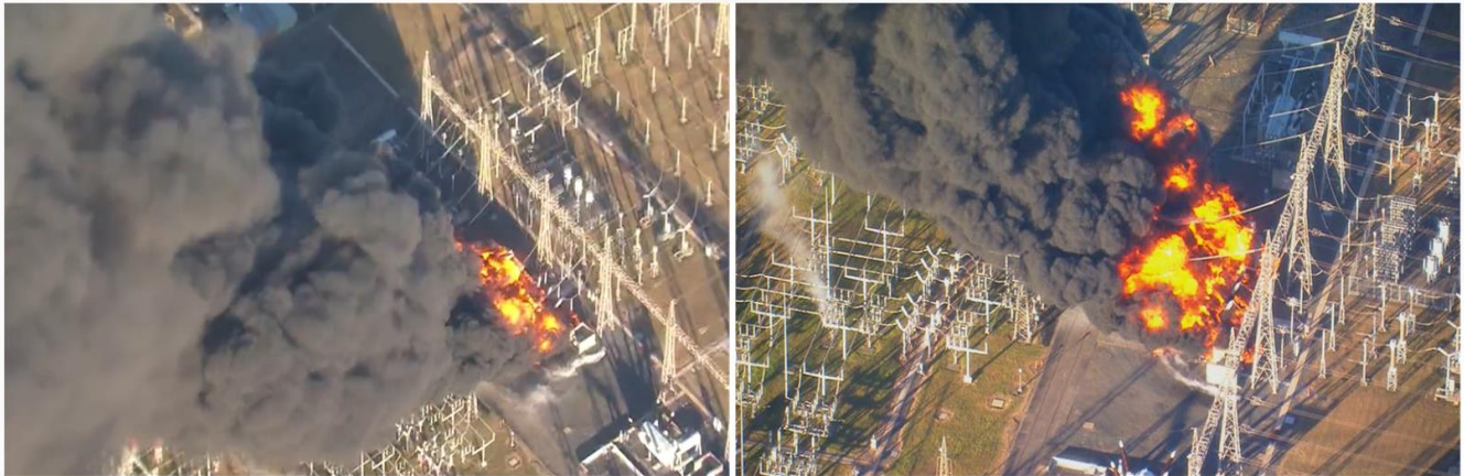
Figure 3: Photos of Dapto Substation fire 7
