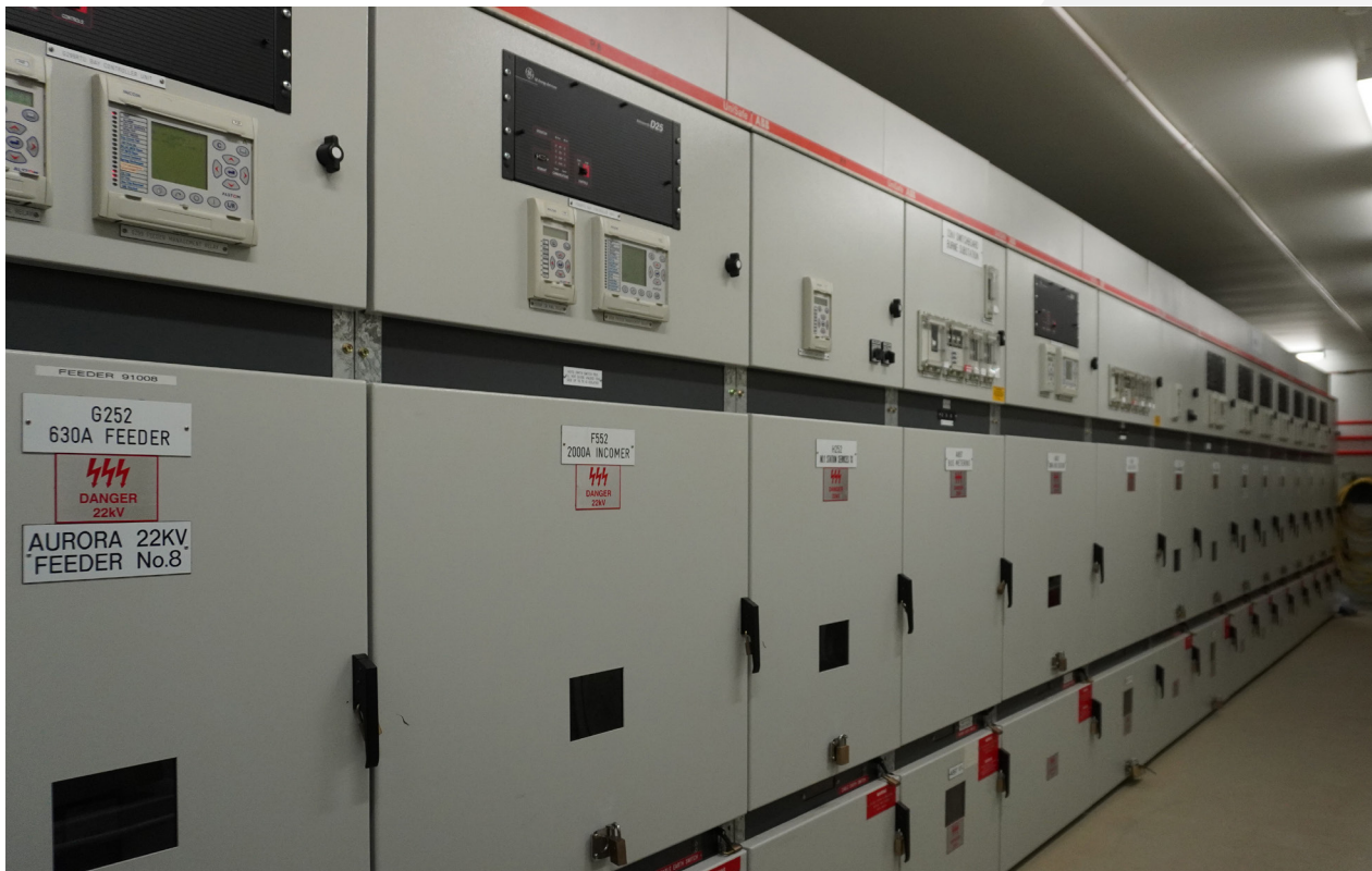
Pictured: Medium voltage distribution equipment
