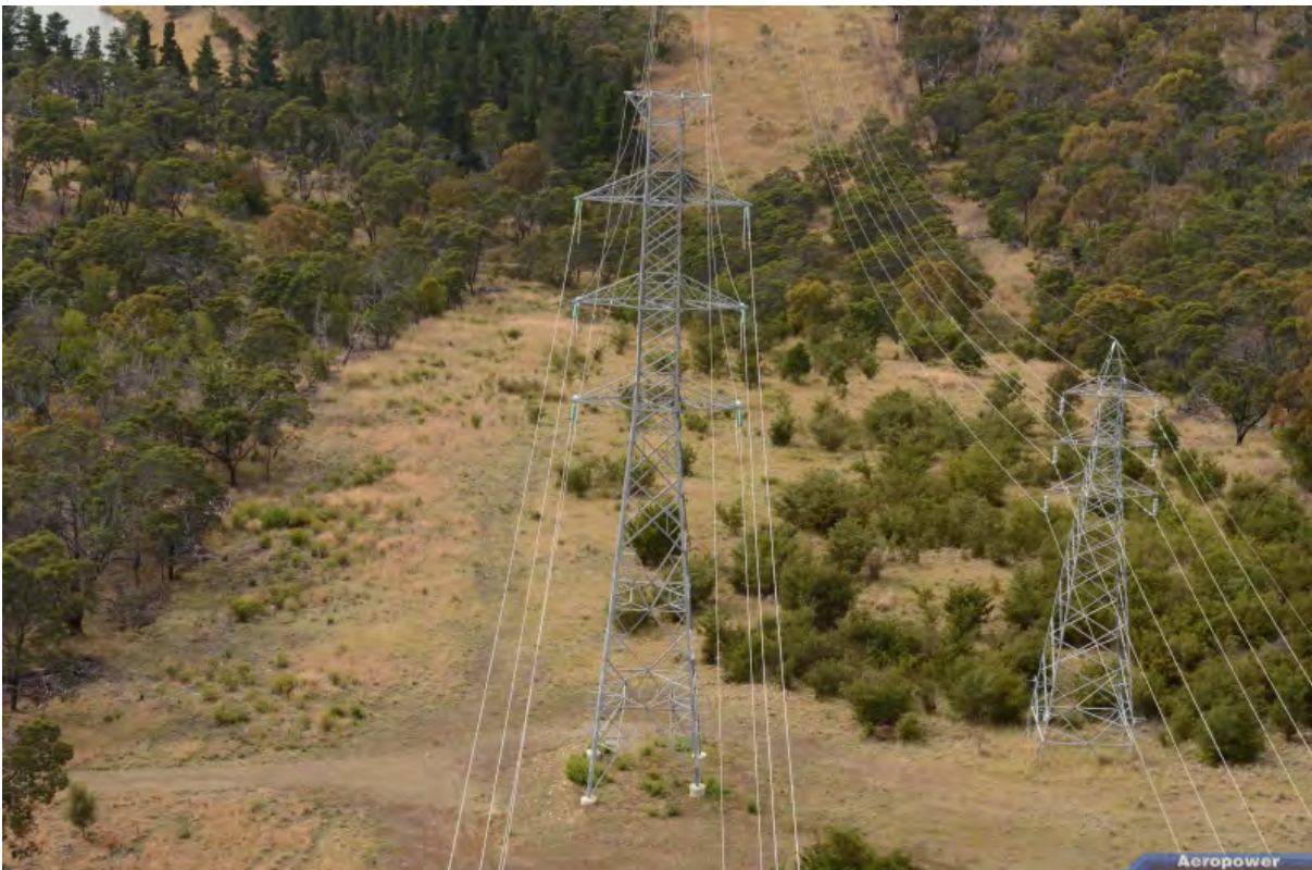
Plate 3-1 Typical double circuit 220 kV transmission tower adjacent to typical double circuit 110 kV transmission tower
