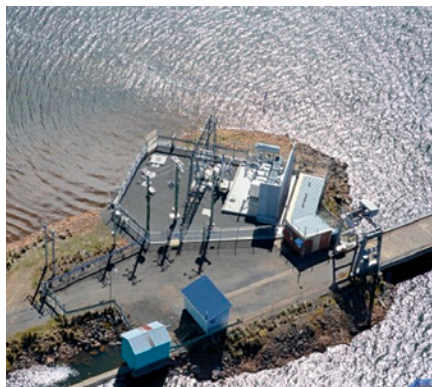
Arthurs Lake Substation
