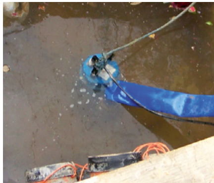
Dewatering pumps must be kept in the clear surface water to prevent pumping bottom sediment Source: Derwent Estuary Program
