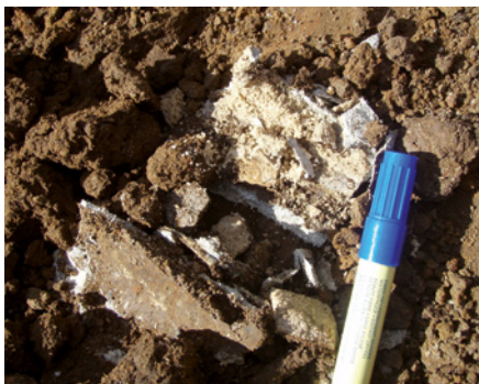
Work should immediately cease if broken asbestos is uncovered
