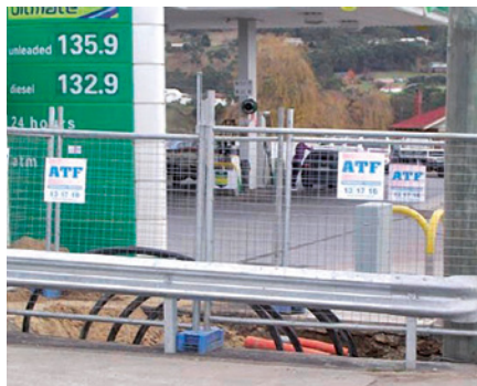
Care should be taken to look out for contaminated soil when working around high risk areas such as service stations
