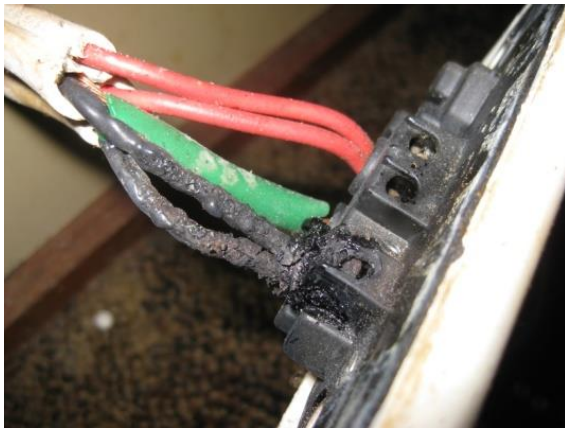
Poor connection and burnt wiring
