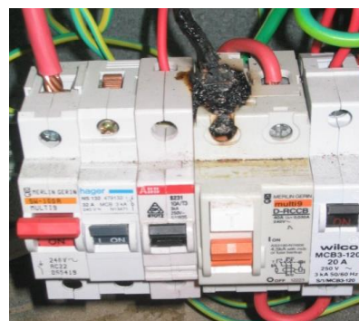
Loose RCD connection
