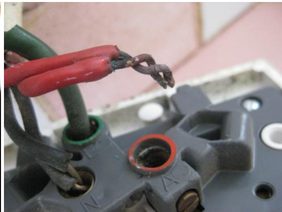
Loose / poor active connection
