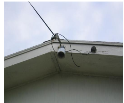
Broken service neutral at POA
