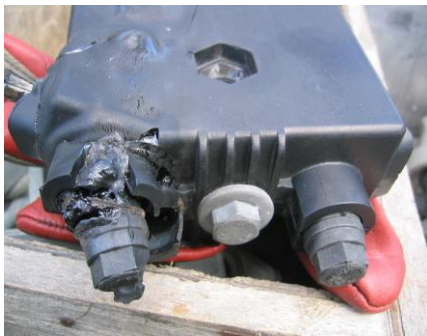
Poor IPC connection
