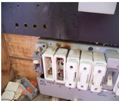
Burnt out fuse
