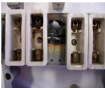
Failed active on federal switchboard
