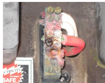
Poor termination / corroded link
