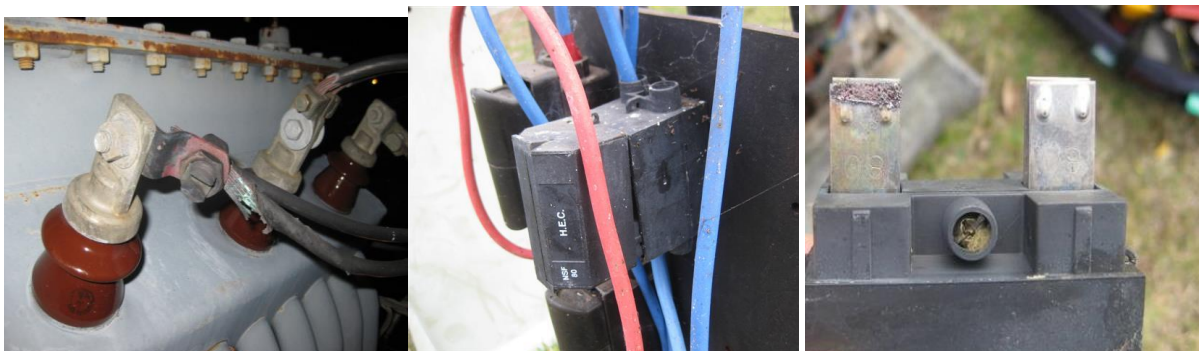
Hot / poor connection at TX
