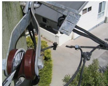
Broken service neutral at pole
