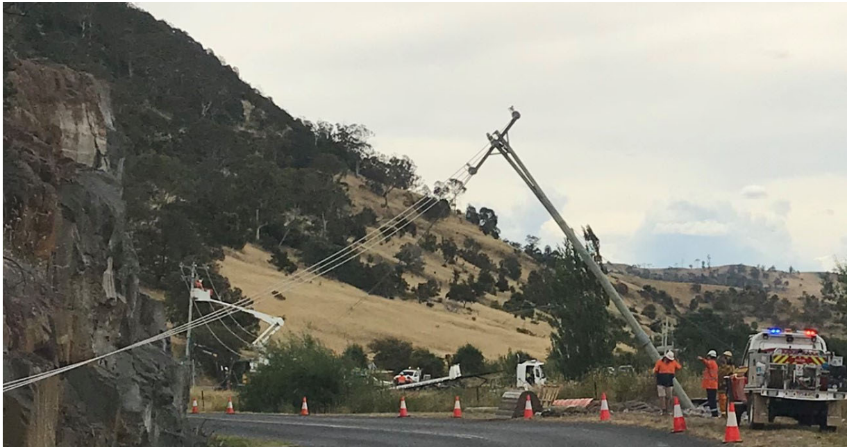
Photo 4: Illustrates split in pole top
