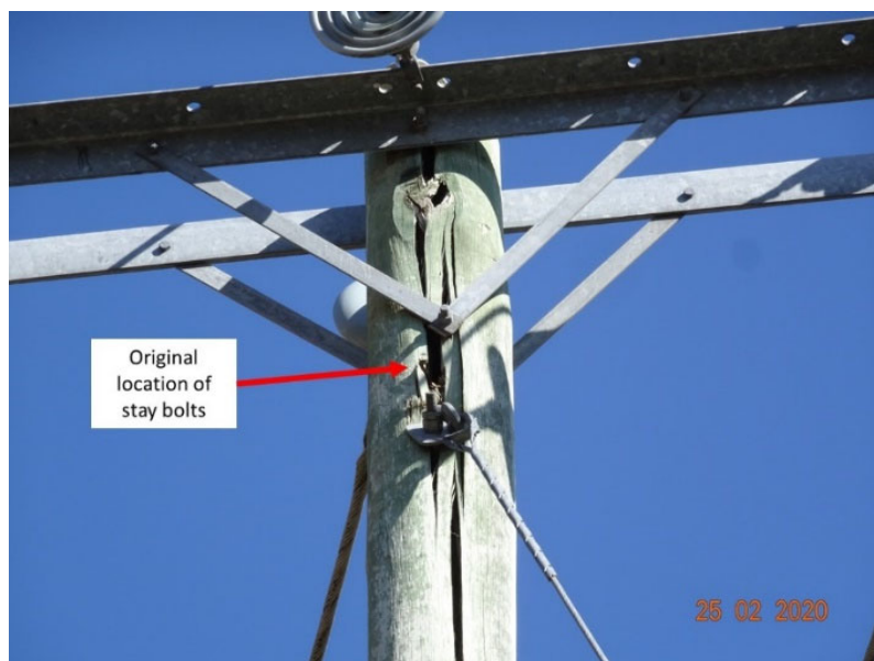
Photo 7: Illustrates crack in pole (taken 25/02/2020)
