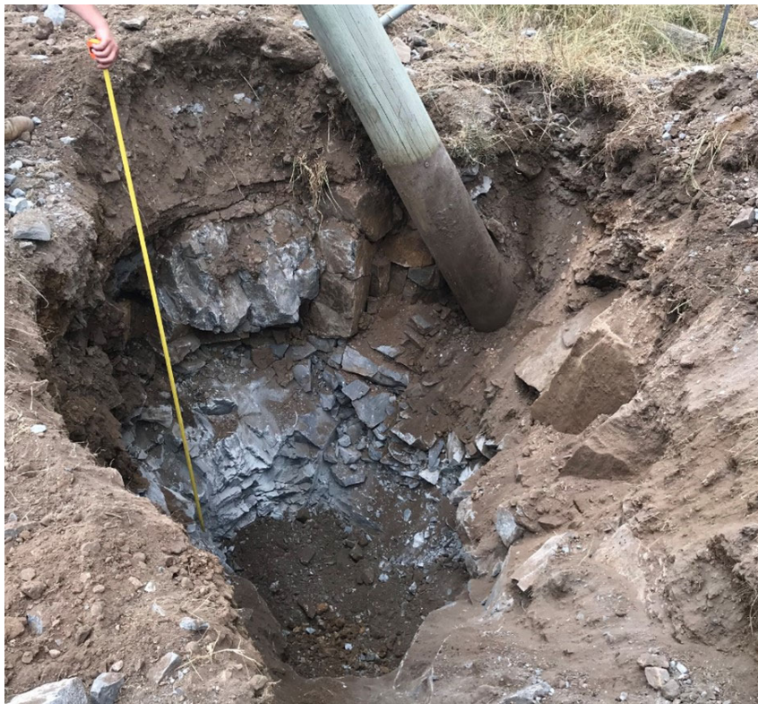
Photo 6: Shows pole foundation compromised between pole and new pole hole (after dig out)
