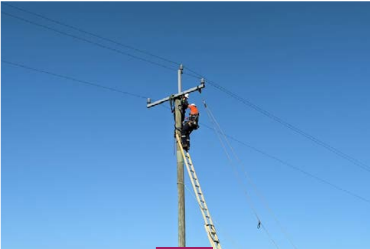
TasNetworks' crew installing a new delta pole top (using fibreglass cross arms) on our distribution network.
